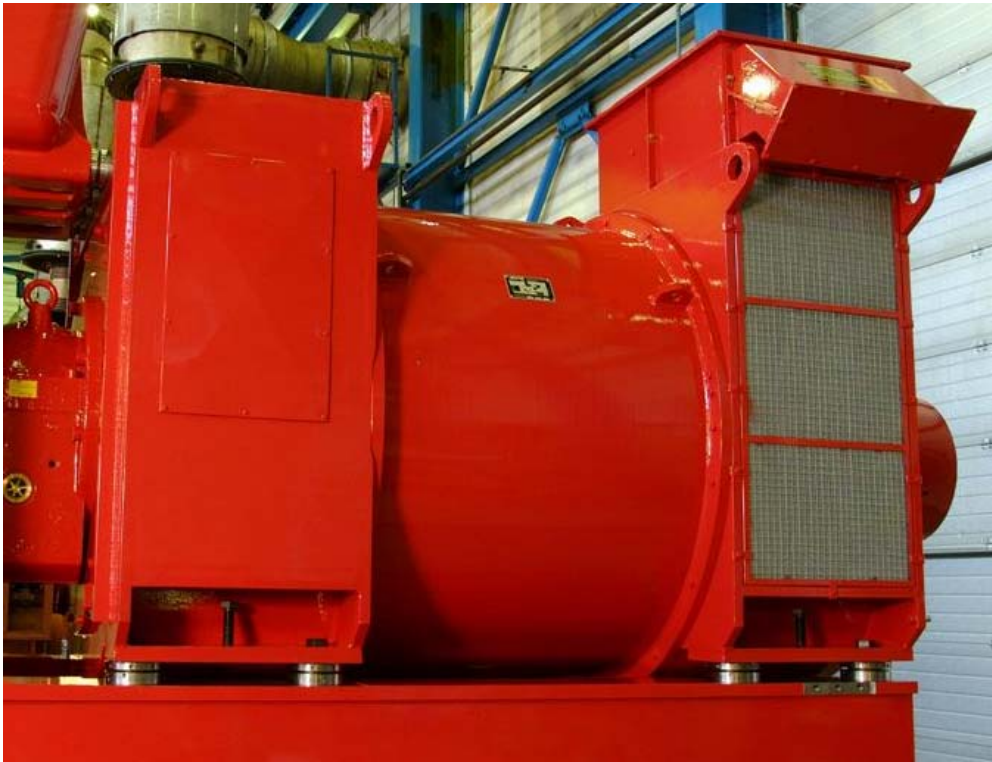
Figure 5.1.6.2 Generator of genset mounted on Vibracon ® chocks.
