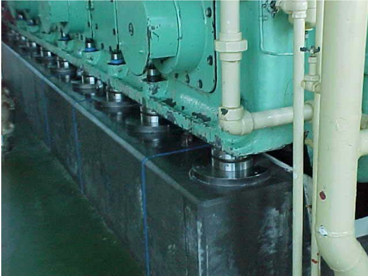
Figure 5.1.6.4 Overview of engine mounted on Vibracon® chocks on a concrete foundation.
